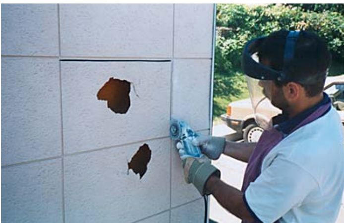
B. Perform vertical cut 1 cm (1/2") inside right side joint of broken panel.
