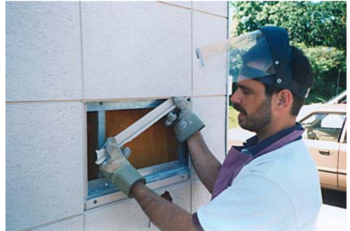
D. With screwdriver and pliers, remove both attachment strip and vertical gutter left in place by breaking them. Be sure to keep in place attachment screws to provide support for replacement panel.
